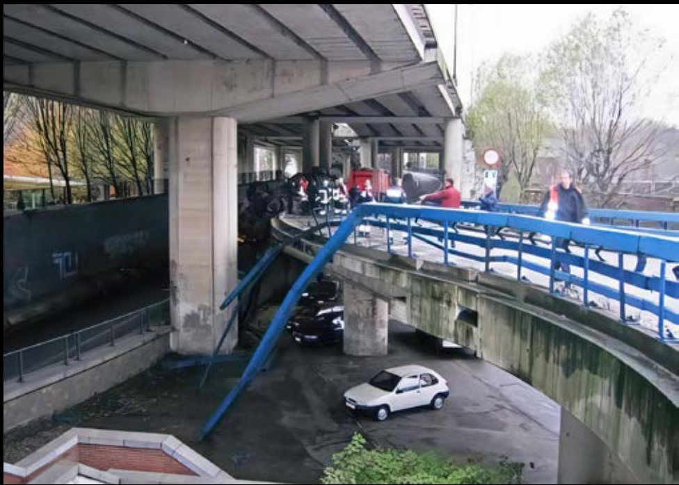
ABOVE: Use of the old style, non-tested, Mailloux parapet design ceased in Belgium following the introduction of the European Standard EN1317.2
