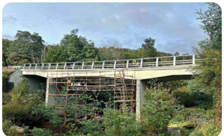
Remediation works on the Ringarooma River bridge near Moorina in north-east Tasmania included bridge strengthening works, application of a new wearing course, and installation of Australia's first DOLRE Regular (TL4) Low Stress Parapet System.
