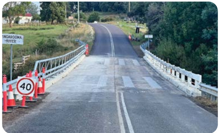
Taken during construction, this image shows the new DOLRE barrier on the left, and the old concrete post and rail barrier on the right-hand side of the bridge deck prior to its removal and replacement.
